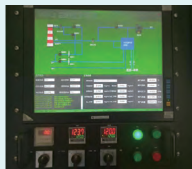
▶ VOCs on-line monitoring system
