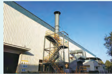
▶ Continuous carburising line fume purification
